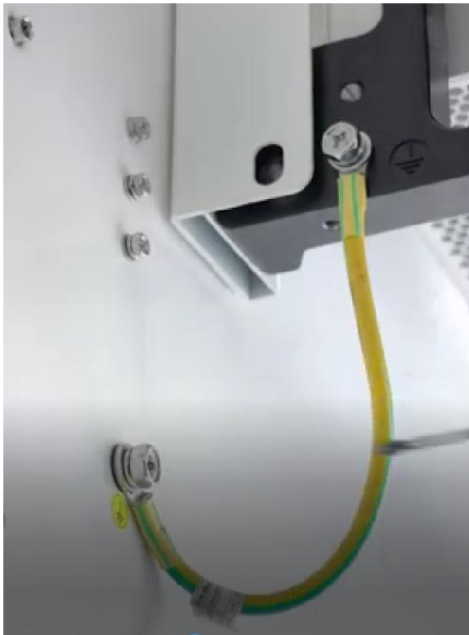
Figure 7-6 Ground connection with cabinet enclosure
