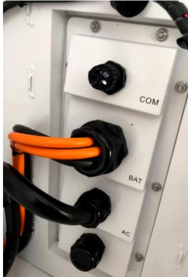
Figure 7- 12 Steps of threading cable
