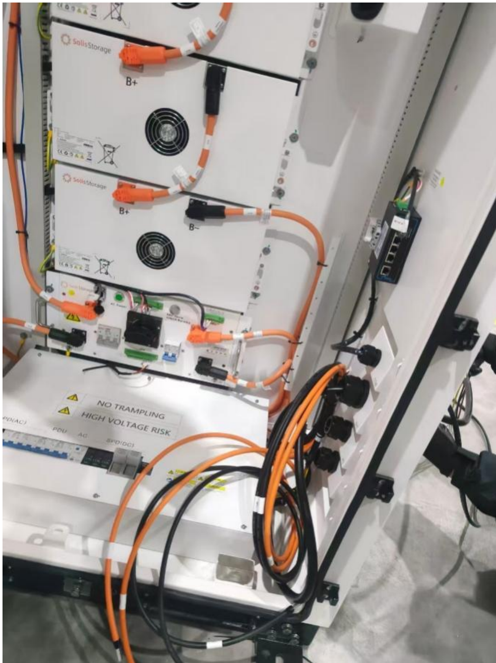
Figure 6- 1 Pre-installed cables inside cabinet
